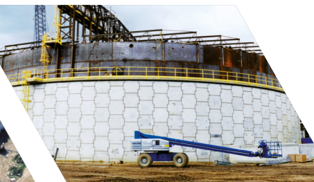
Oil sands separator tanks - Muskeg (Canada)
