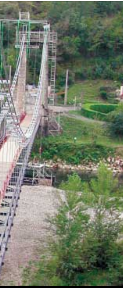
Freyssinet specializes in the repair of suspension bridges, and has developed a method derived from cableways for handling heavy loads over long spans.
