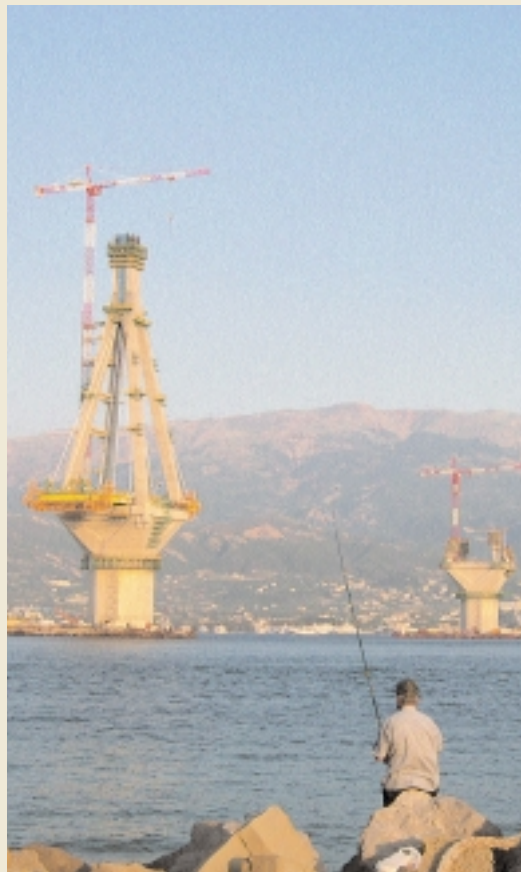
In the seismically active region of Corinth Gulf, soil displacement between two piles may reach 2 m.
